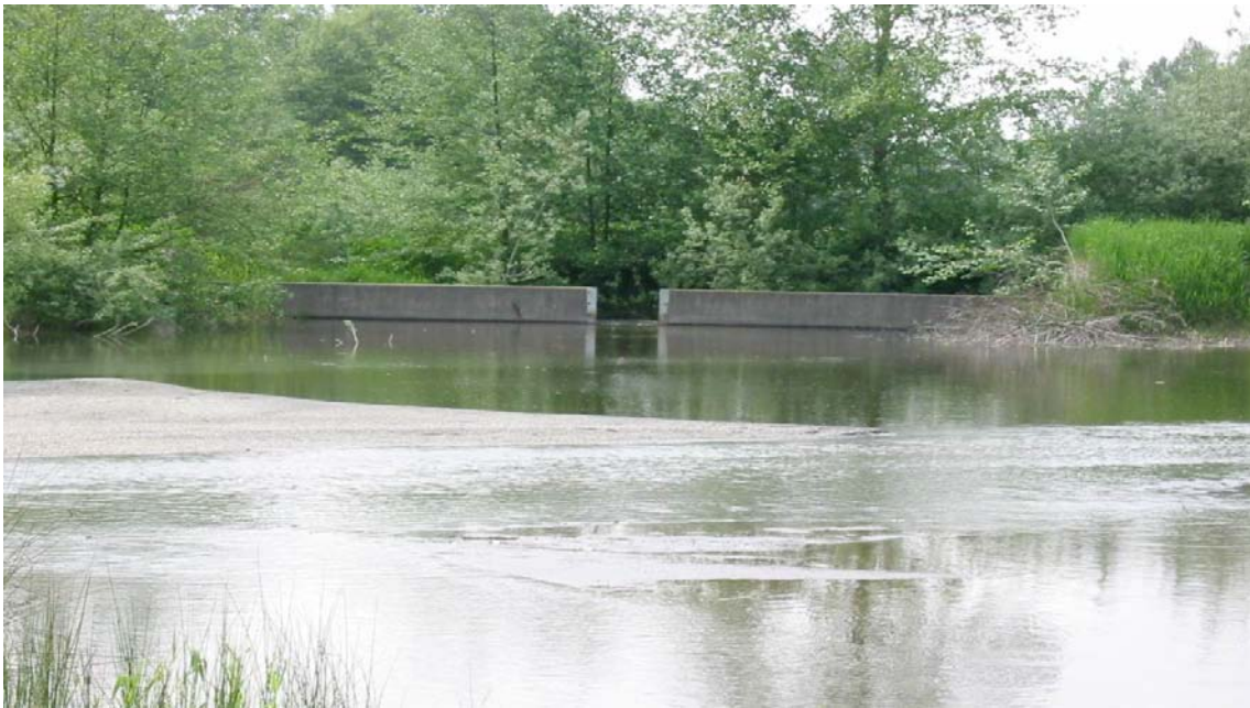
Instream Sediment Detention Basins Figure 2: Coal Creek sediment basin, Skagit County. Looking downstream from basin to slot-type outlet structure. Stream enters on left, deposition shoaling in middle left.
