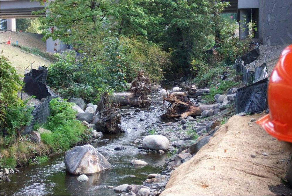
Figure 7. Habitat logs anchored in bank with additional boulder ballast (E. F. Issaquah Ck, I-90 Sunset Interchange, King Co., WA).
