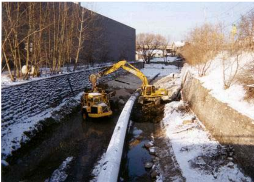
Figure 6. Dewatering an urban stormwater channel in preparation for stream restoration. The Menomenee River is diverted through a pipe, with coffers at each end defining the work area. Note track hoe on temporary in-channel pad. Source: Inter-Fluve, Inc.
