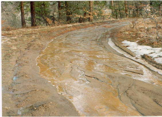
(a) Surface erosion from a road
