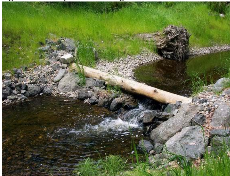
Figure 9. Example of failed log/rock weir.
