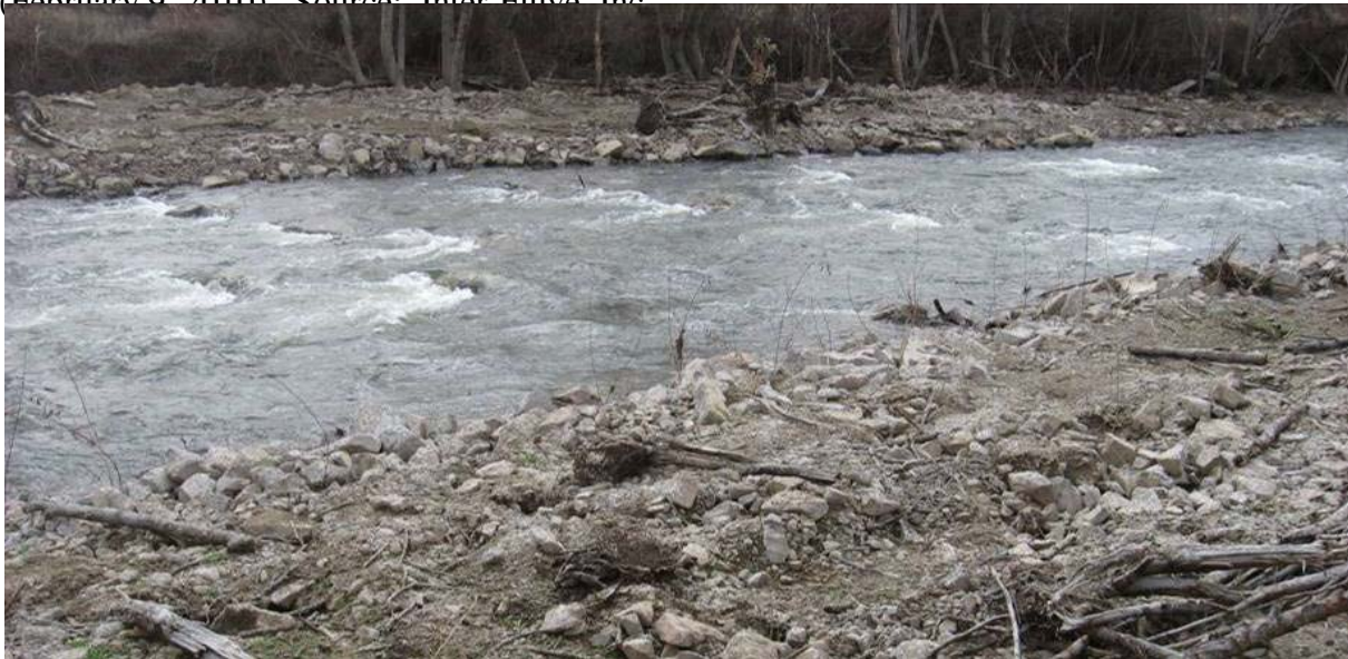
Figure 11. Roughened channel / constructed riffle constructed following dam removal (February 9, 2010) Source: Inter Fluvio, Inc.
