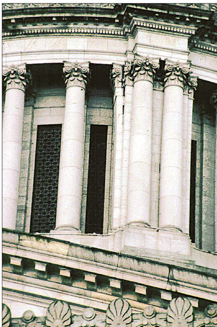
Figure 16. Damaged pilaster on State Capitol building, Olympia.
