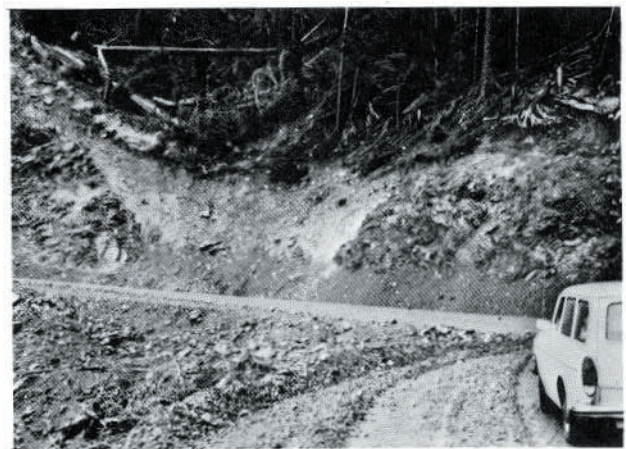
Figure 4—Soil wedge partially filling depression in sedimentary bedrock, western Olympic Peninsula. Note the characteristic “U”-shaped depression and the great soil depth compared to adjacent areas.
