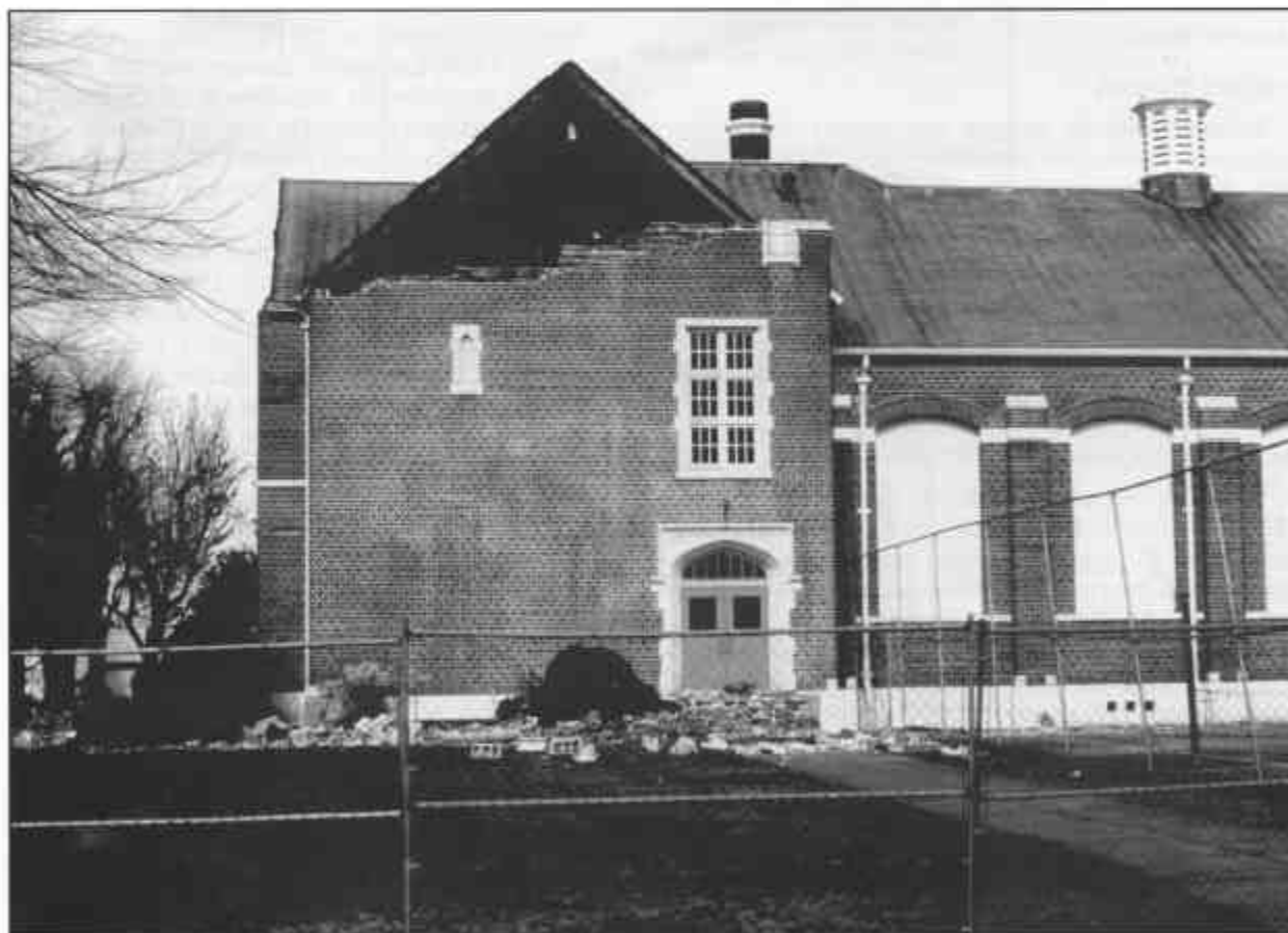
Figure 1. Earthquake damage at Molalla High School from the Scotts Mills ("Spring Break") earthquake, March 25, 1993.
