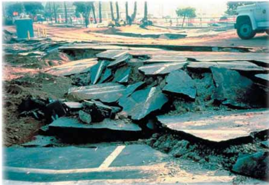
Figure 3. This road was destroyed by liquefaction, when soil turned to liquid during the shaking of the ground. Many soils in the Seattle area can liquefy, including those in the Kent and Duwamish Valleys.
