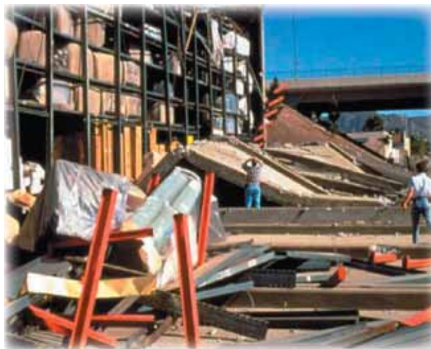
Figure 2. Many warehouse buildings are tilt-ups, which often don't fare well in earthquakes. The destruction of even one wall can cause injuries, leave inventory vulnerable, and create rubble on parking lots and streets that impedes rescue and recovery efforts.
