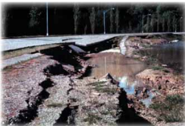
Figure 1. Road damage like that from the 1965 Olympia earthquake could make it difficult to resupply many businesses throughout Puget Sound.
