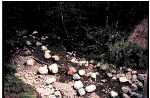
Boulder Clusters Figure 5: Constructed boulder clusters in Lynch Creek, King County, Washington
