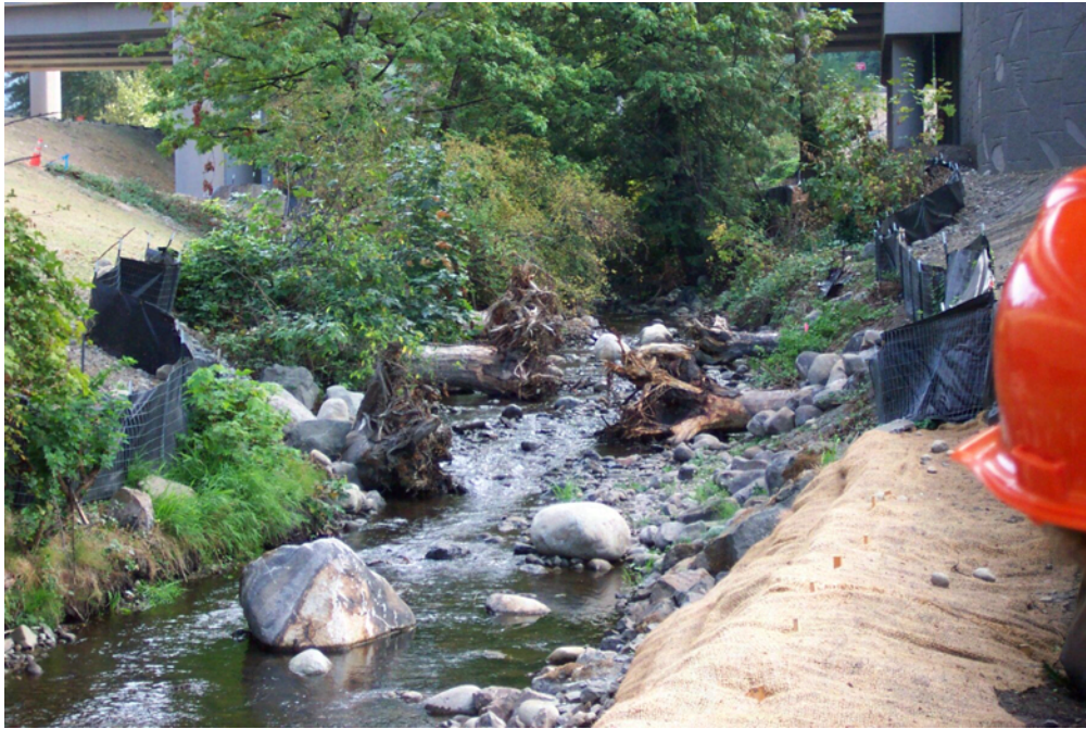
Figure 4 E. F. Issaquah Ck, I90 Sunset interchange, King Co., habitat logs anchored in bank with additional boulder ballast.
