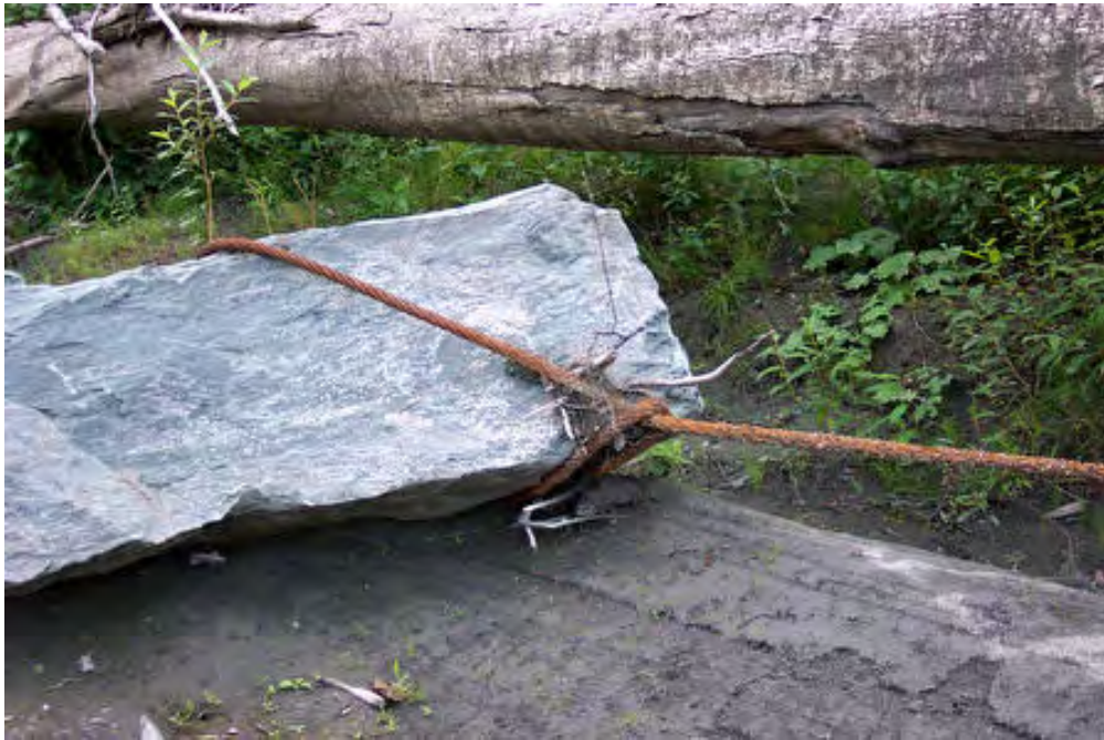
Figure 6 Boulder anchor. Cable should be protected from abrasion with hydraulic hose or similar protection.
