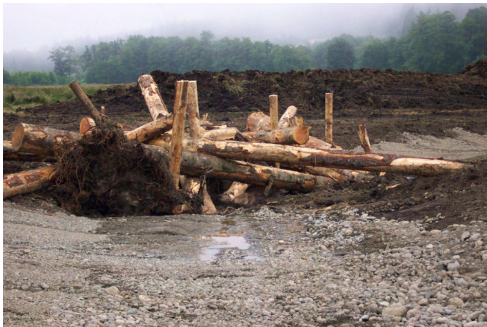
Figure 5 Salmon Ck, Jefferson Co., channel restoration project. Piling used to increase stability of log jam.
