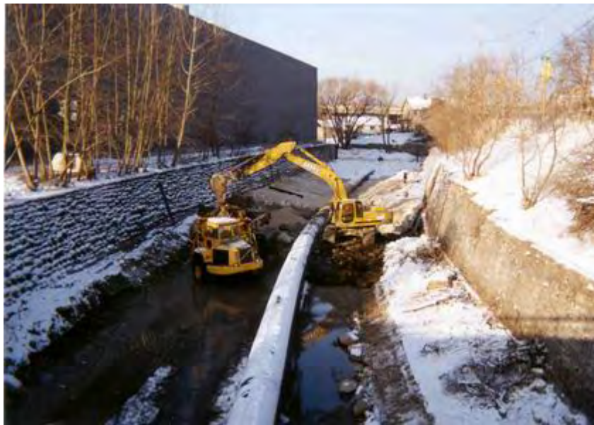
Construction Considerations Figure 6. Dewatering an urban stormwater channel in preparation for stream restoration. The Menomenee River is diverted through a pipe, with cofferdams at each end defining the work area. Note track hoe on temporary in-channel pad.
