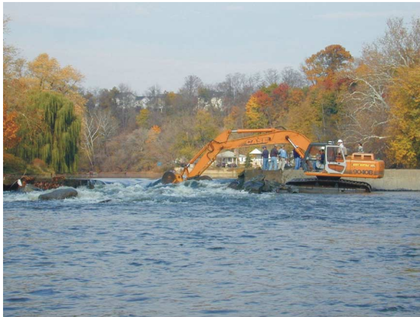
Fig. 7. A power shovel operating in the removal of a typical low-head, run-of-river dam: Waterworks Dam on the Baraboo River, Wisc., 1997. Photo courtesy of the River Alliance of Wisconsin.
