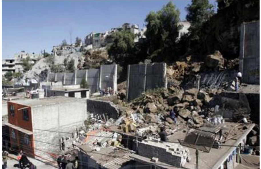
Figure C36. Caution is required in locating and constructing debris-flow retaining walls. This is a photograph of the partial failure of a retaining wall, caused by a landslide in Iztapalapa, a suburb of Mexico City, Mexico. The landslide slid onto a house at the toe of the slope, killing two people, and was triggered by heavy rains in the area. The house was below the 5-meter-high (15 yards) wall, but the wall could not withstand the mass of rocks and soil. (Photograph by Chinagate/Xinhua.)
