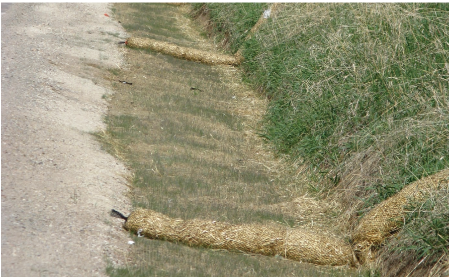
Figure C11. Straw wattles on the side of a road capture sediment and hold it onsite, enabling seeds to settle and germinate, aiding the revegetation process. (Photograph by Lynn Highland, U.S. Geological Survey.)
