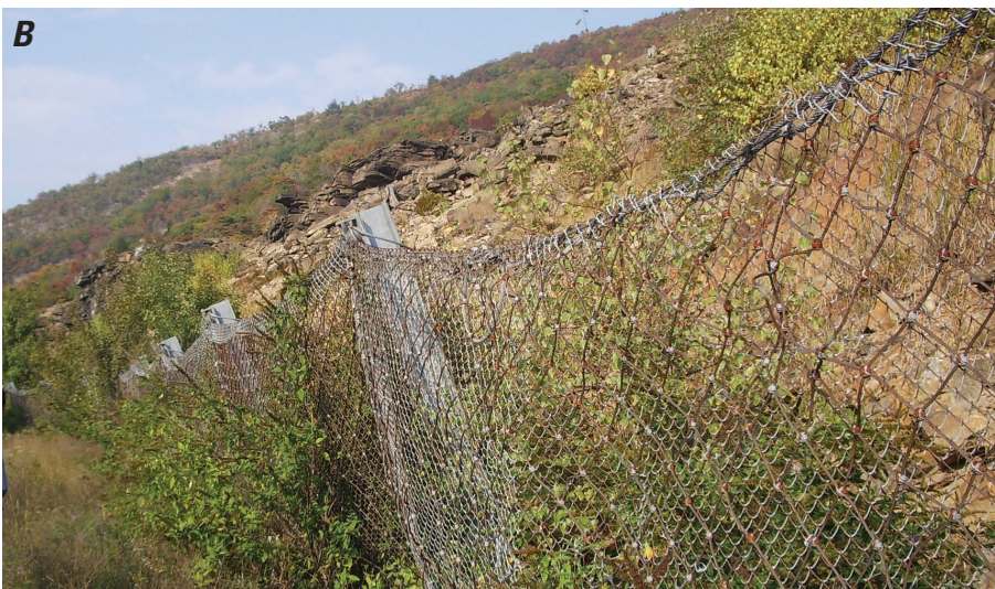
Figure C22. Protective rock barrier fencing along (A) a dirt trail in Pennsylvania, USA, and (B) a roadway in coastal California, USA. (Trail photograph, Lynn Highland, U.S. Geological Survey; roadway photograph from Federal Highway Administration, USA.)
