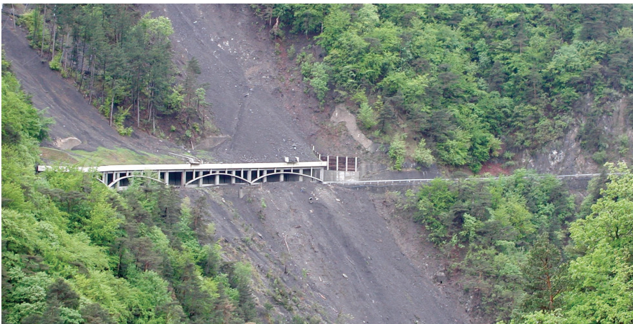
Figure C26. A rock avalanche shelter in the Montenyard area of France. The length of the shelter may be insufficient as a debris flow has damaged the road, shown to the right of the shelter. (Photograph by Dave Giles Engineering Geology Consultancy Group, University of Portsmouth, United Kingdom.)
