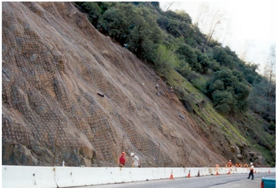
Figure C21. Example of wire mesh placed over a rocky slope to contain the rocks that may come down.
