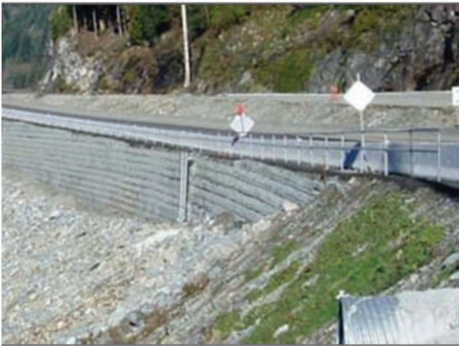
Figure C5. Schematic and photograph of a rockfill buttress in Canada. (Graphic is from Reference 11.)
