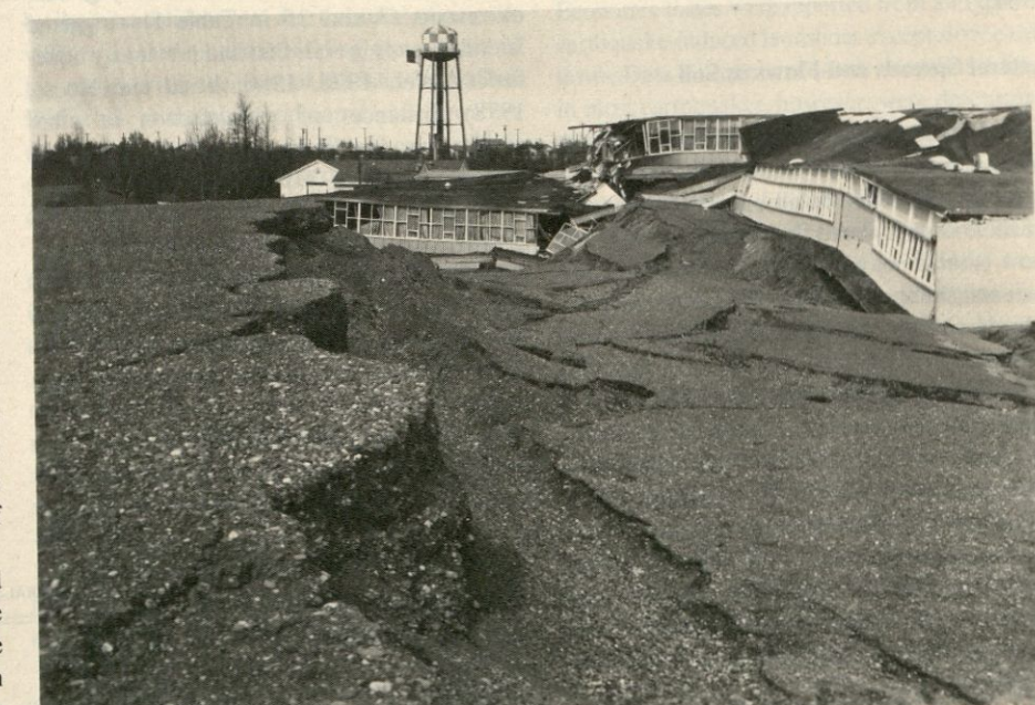
Figure 7. Elementary school destroyed by the Government Hill slide in Anchorage, Alaska. One wing of school dropped into graben at head of slide. Slide triggered by the 1964 Alaska earthquake (16 in Table 1). Photograph from Hansen (1966).
