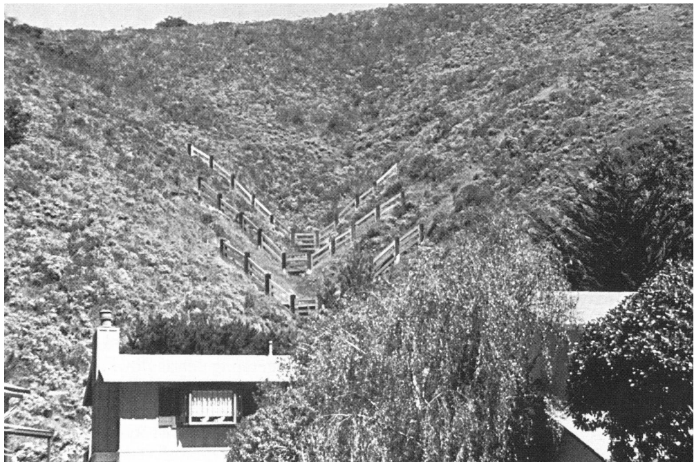
Figure 28. Debris fences installed below potential initiation sites in Pacifica, California. (From Montgomery and others, 1991)
