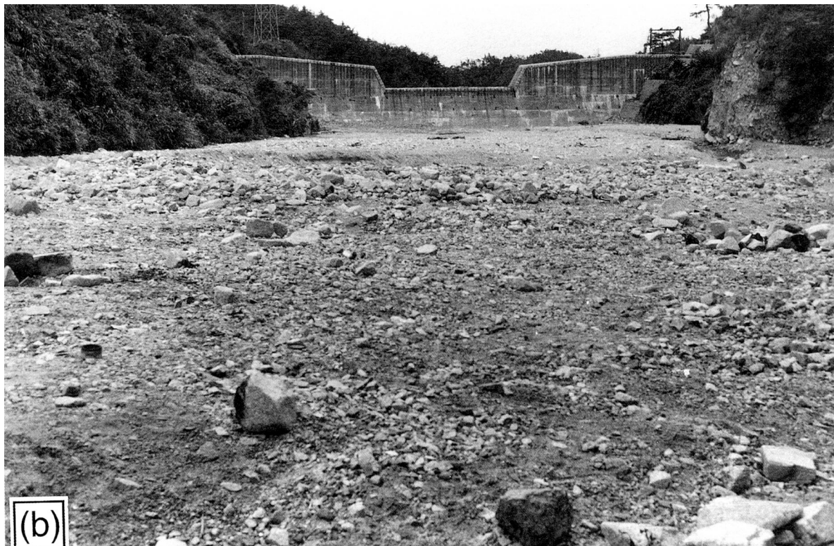
Figure 33. Check dam in Hyogo, Japan (30 m high, 78 m long, storage capacity 300,000 m 3 ), (a) before and (b) after a debris flow. (Photo from United Nations, 1996)
