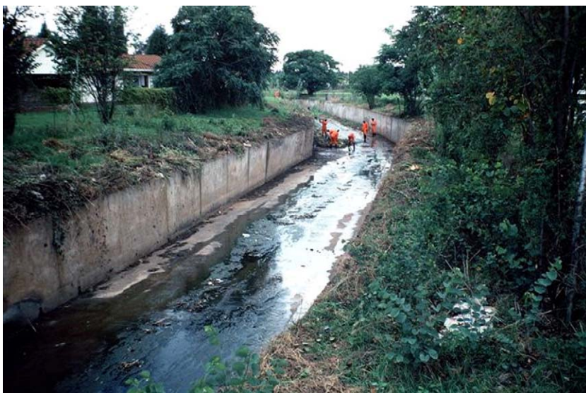
Fig. 7. Avondale Stream in Harare, Zimbabwe, illustrating how artificial manipulation of urban streams commonly results in reduced sinuosities (see Whitlow and Gregory, 1989; photograph by K.J. Gregory).
