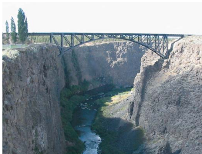
Figure 2. The Crooked River Gorge looking west from the old US 97 Bridge at Peter Skene Ogden State Park. Note the spring system at the base of the canyon beyond the railroad bridge.
