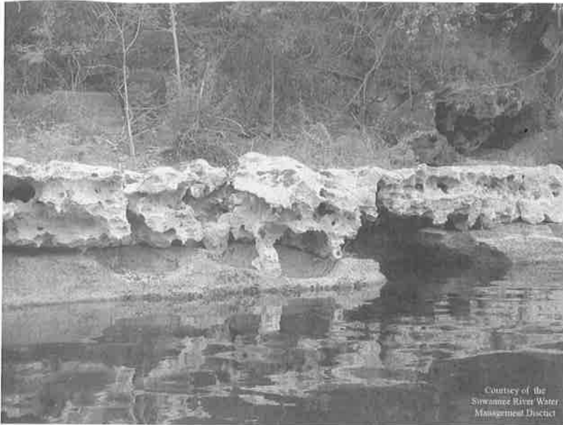
FIG. 4.3 This picture shows an example of limestone dissolution. The location is along the Suwannee River in northern Florida.
