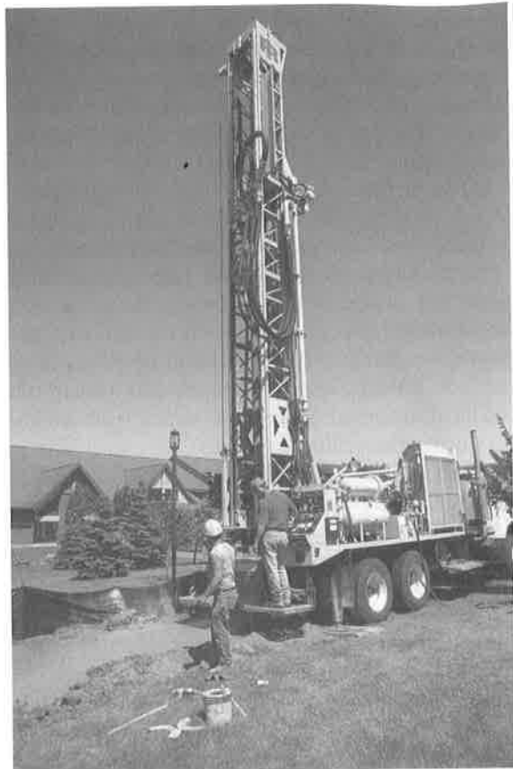
FIG. 4.17 Well-drilling rigs like this one are used around the world to tap precious groundwater supplies. Well drillers can use rotary drill bits, percussion bits that smash rock, or large auger bits if the ground is relatively soft.
