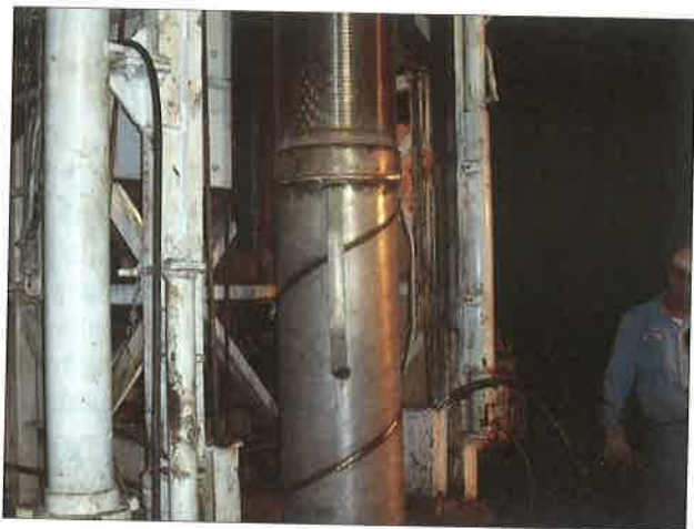
Figure 10.19. Centralizer on a screen (Clear Creek Associates).
