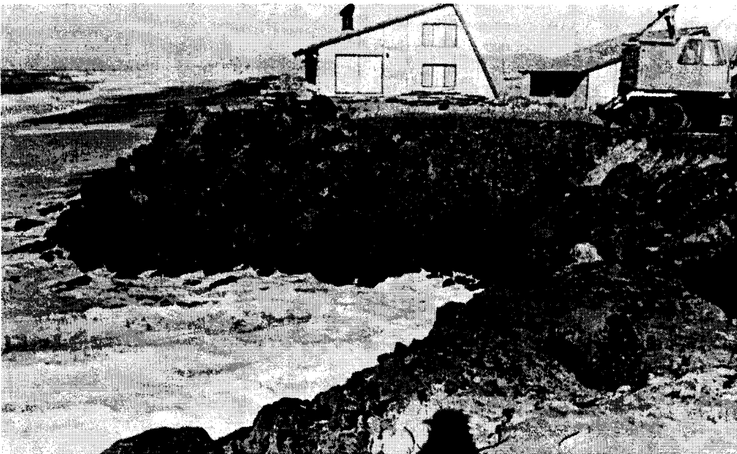
Photo 64. Close-up showing house on left side of above photo where riprap placed earlier at front of house was not sufficient to withstand later storms. Erosion continued to remove sand exposed at either end, requiring additional riprap.
