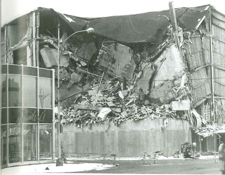
FIGURE 8.19 Comparing Damage to Structures The poorly designed five-story JCPenney building in Anchorage, Alaska, sustained extensive damage. The steel-frame adjacent building incurred very little structural damage. (Courtesy of NOAA)
